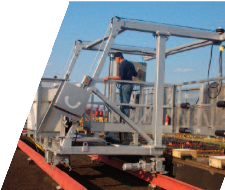
Stick Built - Retrofit
